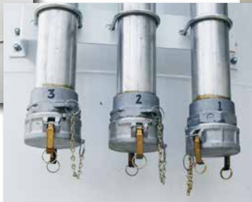
Numbered loading connections
